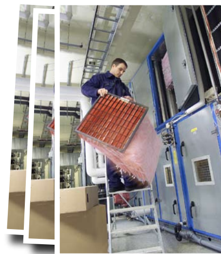
Air filter in air handling unit.
